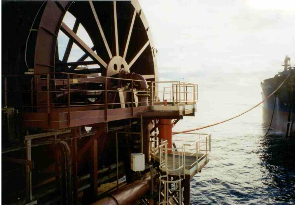
Offloading hose reel at stern of FPSO
