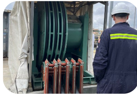
Cable tension and movement monitoring.
